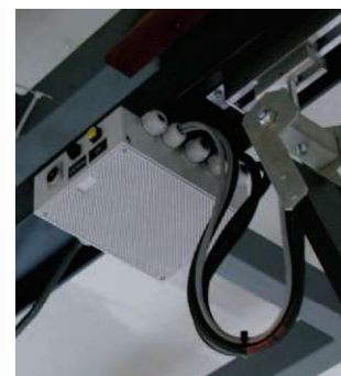
Terminal box (ceiling)
