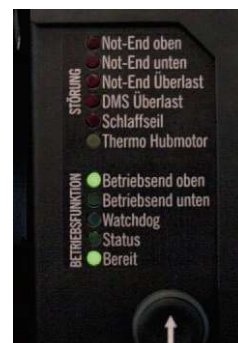
Control switches and status indicators
